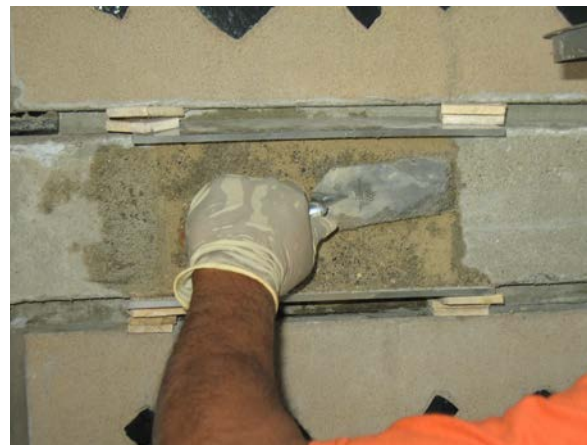
Figure 4. Aggregate was applied to the surfaces of the concrete patches to match the color and texture of the adjacent aged concrete.
