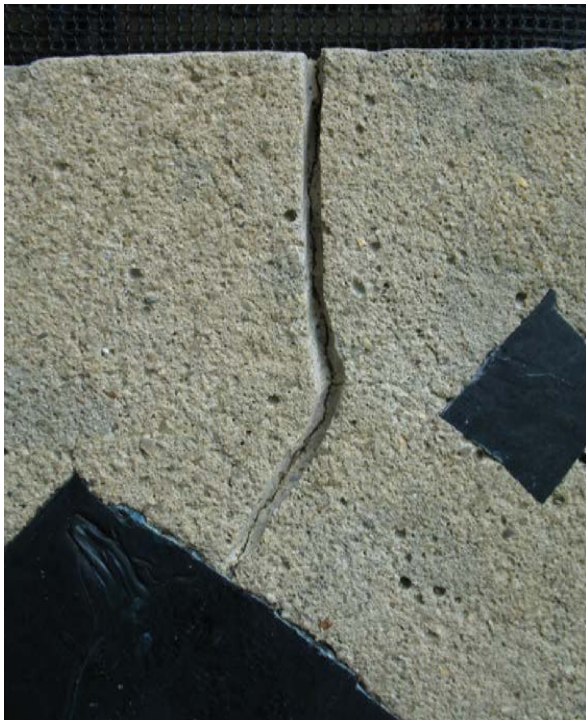
Figure 5. Crack in dalle-de-verre panel routed with diamond tipped dremel blade in preparation for patch installation.
