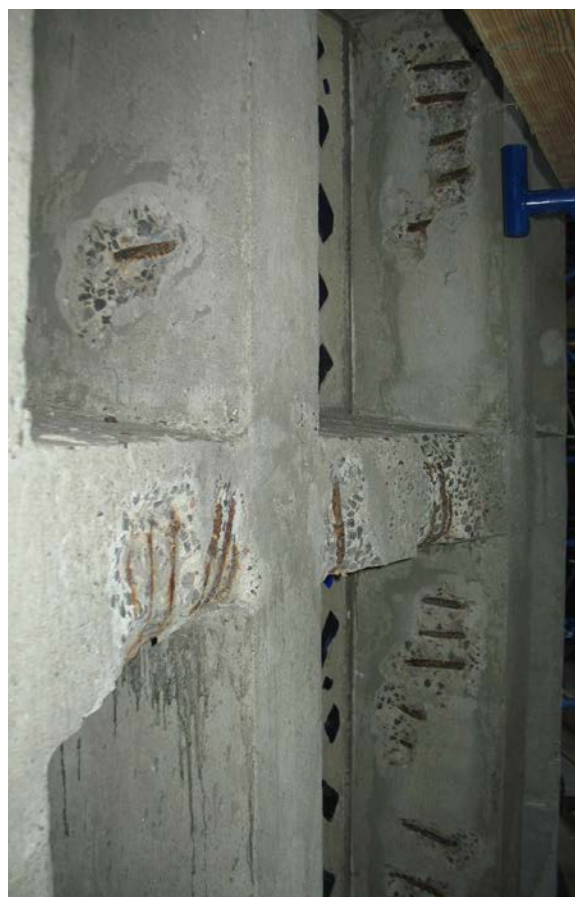
Figure 3. Coffered-side of freestanding wall. Shallowly embedded, corroded steel reinforcing bar exposed by spalling concrete and previous patches.
